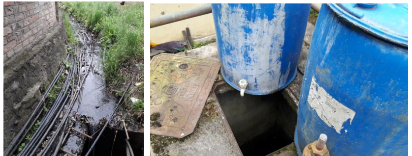
Figure 13: pipelines laid out through storm water drain and abandoned chlorination tank
