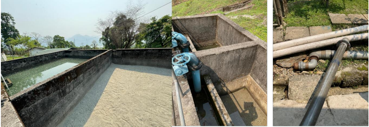
Figure 1 Filtration system not used for treatment (due to blockage) and by passed
