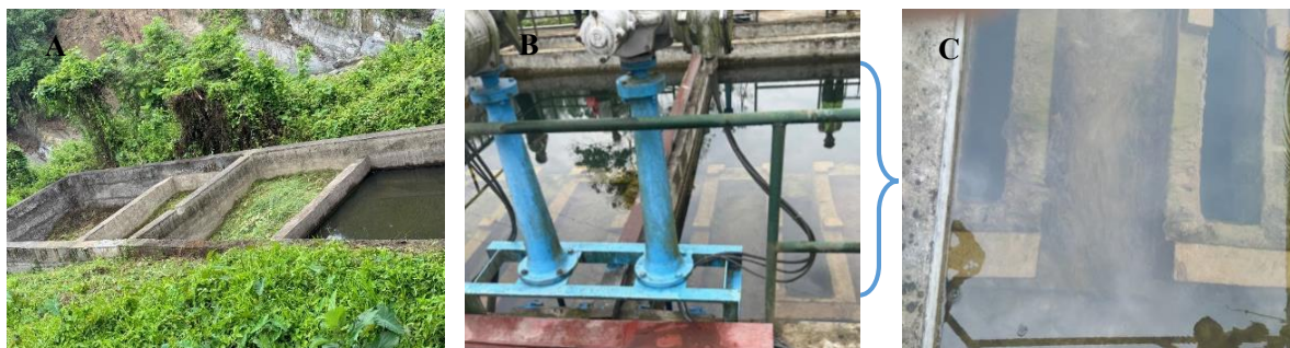
Figure 3 Treatment plant not properly cleaned and maintained (A. Backup treatment plant not properly maintained, B. Open treatment system with high risk of contamination and C. Algae growth inside treatment plant)
