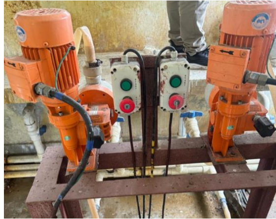
Figure 2 Non-functional equipment for water treatment (Chlorine dosing pumps)
